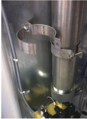
Figure 52 - Right Dryer Column
