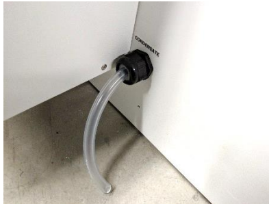
Figure 27 - Power Supply condensate drain
