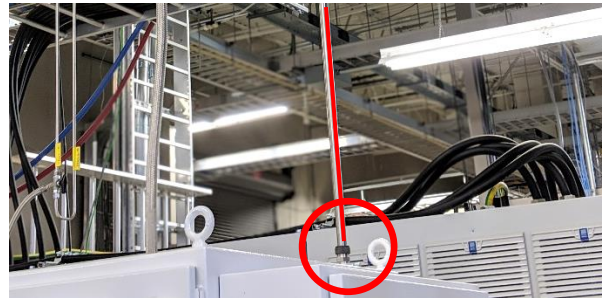
Figure 20 - O2 vent bulkhead passthrough (external)
