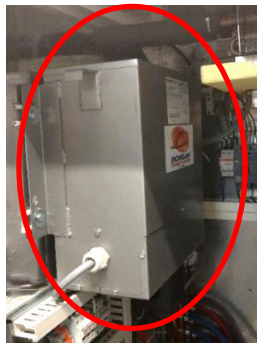
Figure 15 - 380/400/415/480 to 240 Transformer (TXFM1)
