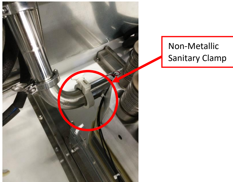
Figure 56 - Cell Stack Return and Hydrogen Product Connections
