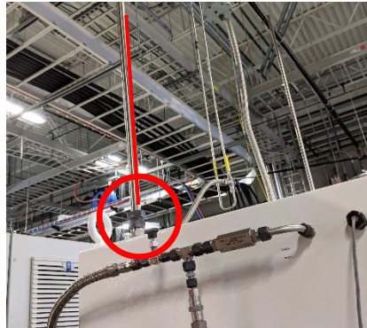
Figure 18 - H 2 vent bulkhead passthrough (external)
