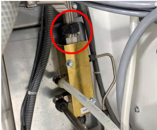
Figure 19 - O2 vent manifold connection (inside)
