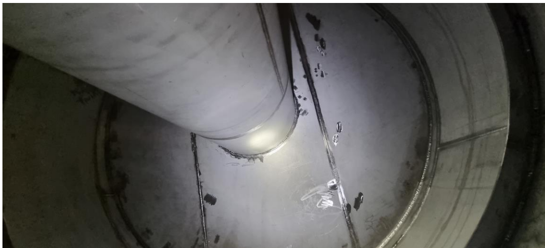
Section 682B.1 Performed internal visual inspection before the final test. The visual appearance of base metal and welding is satisfactory. Internal cleaning is ok.
