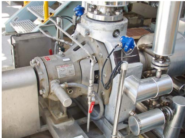
Wilfley pump with thermowells, vibration monitor, steam jacketed case
