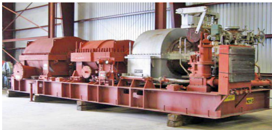
Photo Above: Complete 101 Air Compressor Train
